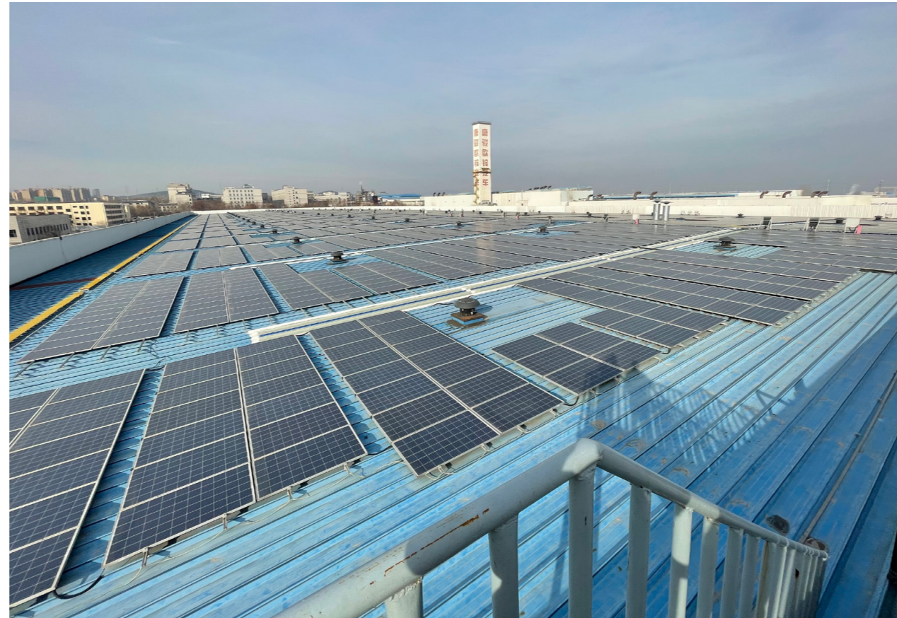
▲ Photovoltaic panels laid on the roof of the workshop and parking area in Tangjun Base of Geely Commercial Vehicle
